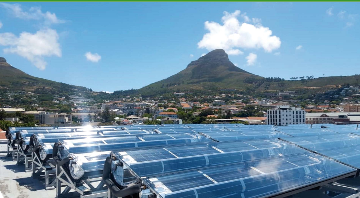
Concentrating PVT system for the Hilton Hotel, Cape Town South Africa: 103 kW th and 17kW peak combined with 4 x 44 kW heat pumps.
