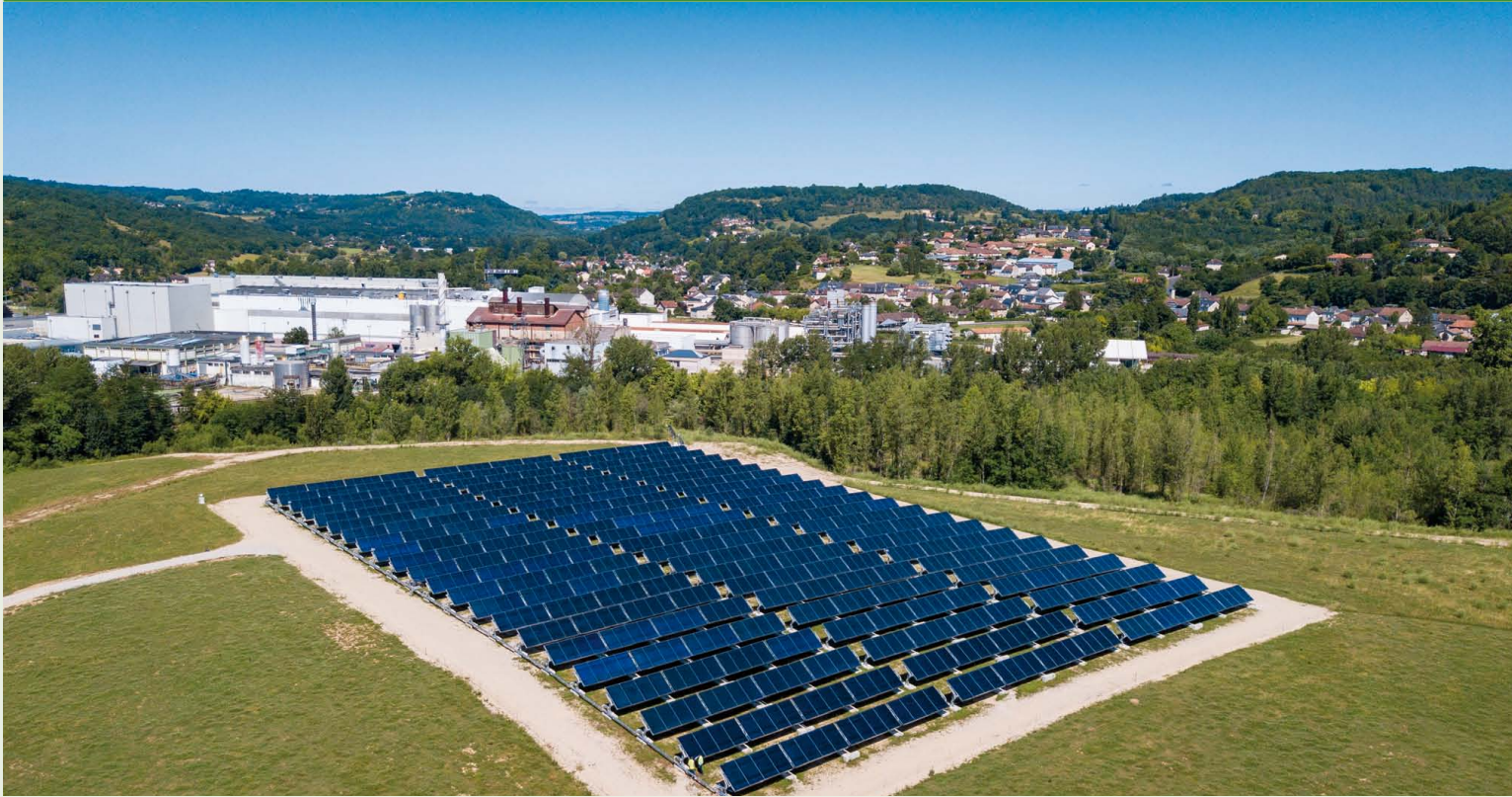
2.9 MW th flat plate collectors on trackers provide heat for the CONDAT Paper Mill in France
