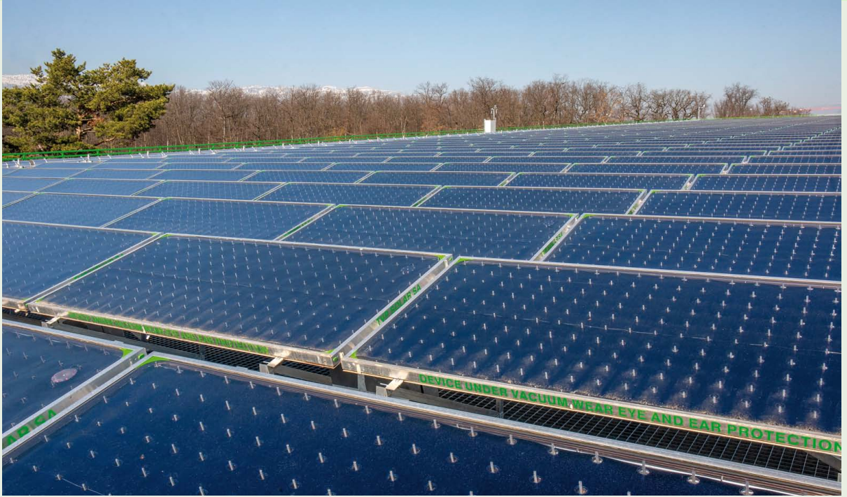
The Swiss solar district heating system in Geneva, with a capacity of 0.5 \text{ MW}_{\text{th}} , is equipped with high-vacuum flat plate collectors and began operation in December 2020.
