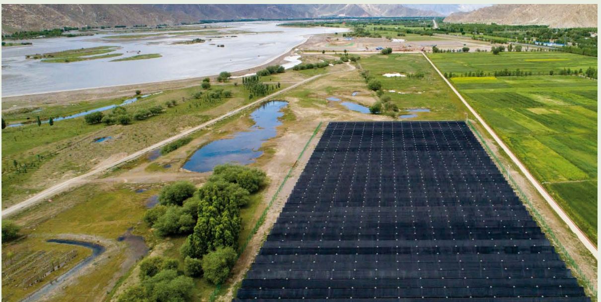
Lasha solar district heating system in Tibet, China with 13,000 \text{ m}^2 collector area ( 9.1 \text{ MW}_{\text{th}} ). Photo: Solareast Holding Company Ltd.
