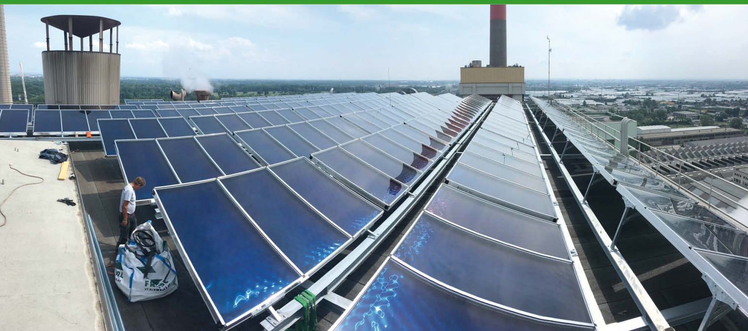
Large-scale flat plate collectors for an industrial application in Vienna, Austria.
