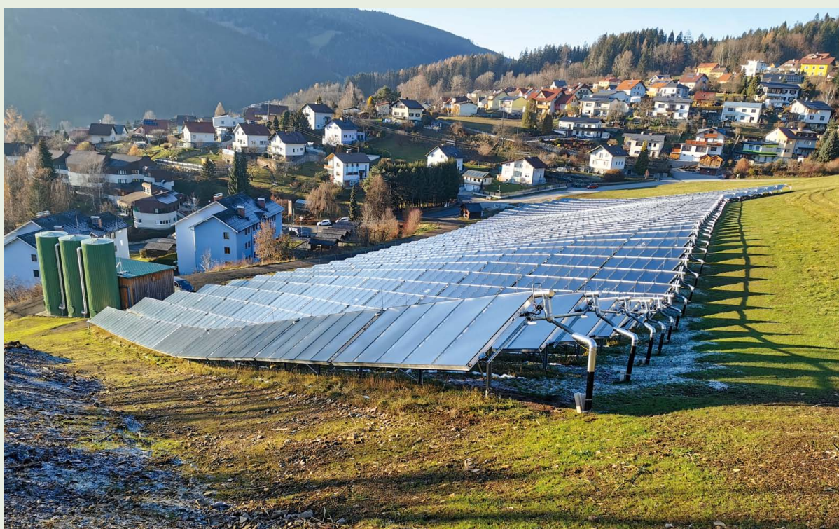
Solar district heating system Müzzuslag, Austria
