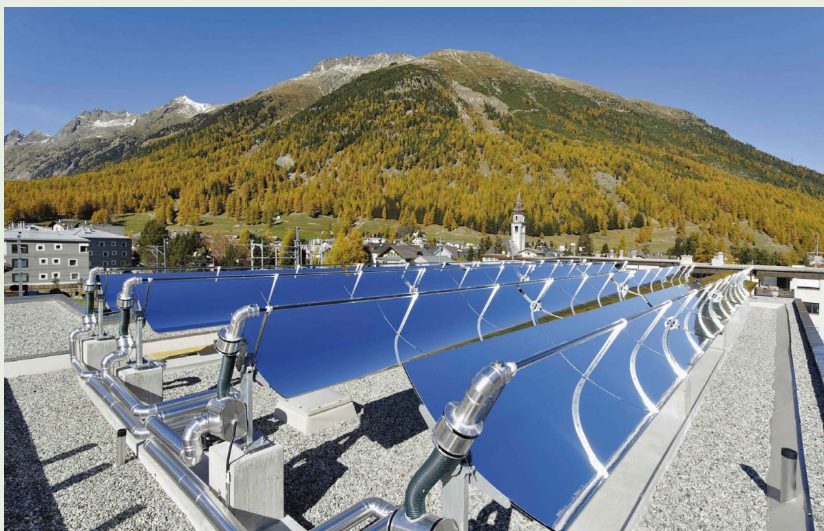
Lataria-Engiadinaisa-Dairy, Switzerland with 115 m 2 of parabolic trough collectors
